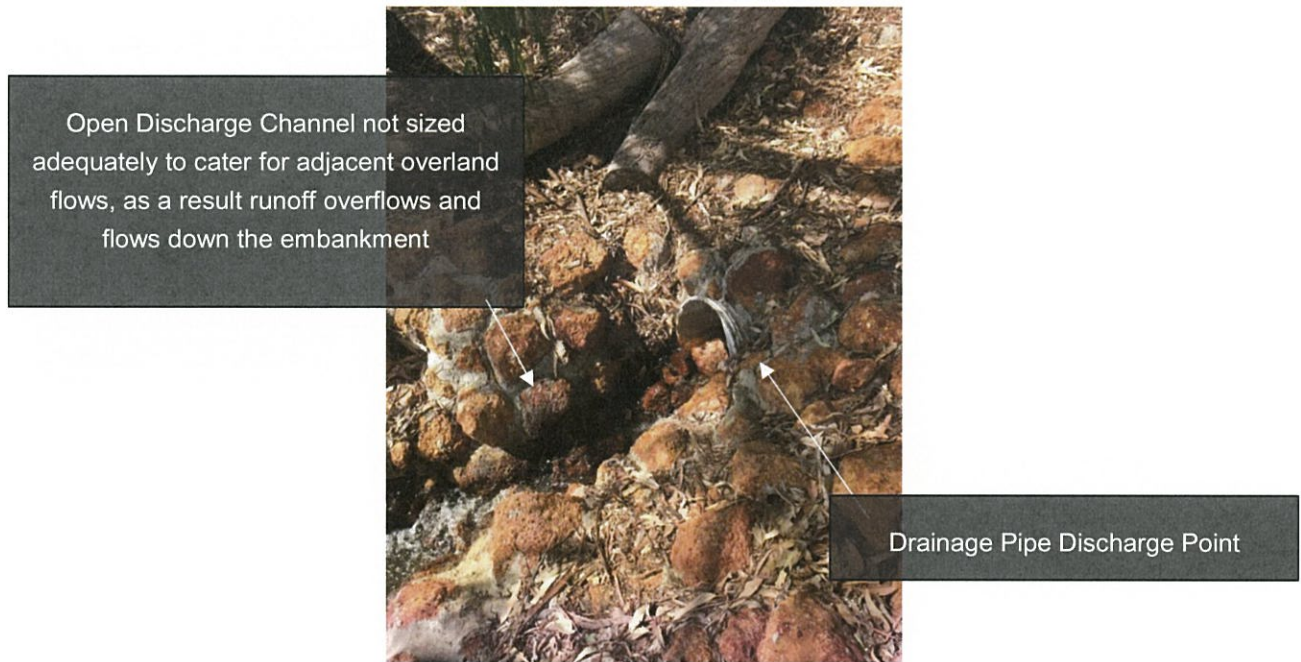
Figure 10 Pipe Discharge Open Channel
