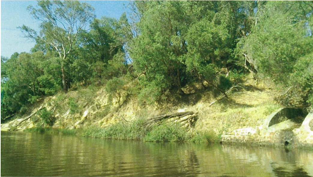
Photograph 5: (Right) Outflow structure. (Left) Recent collapse of several trees due to ongoing slope instability.
