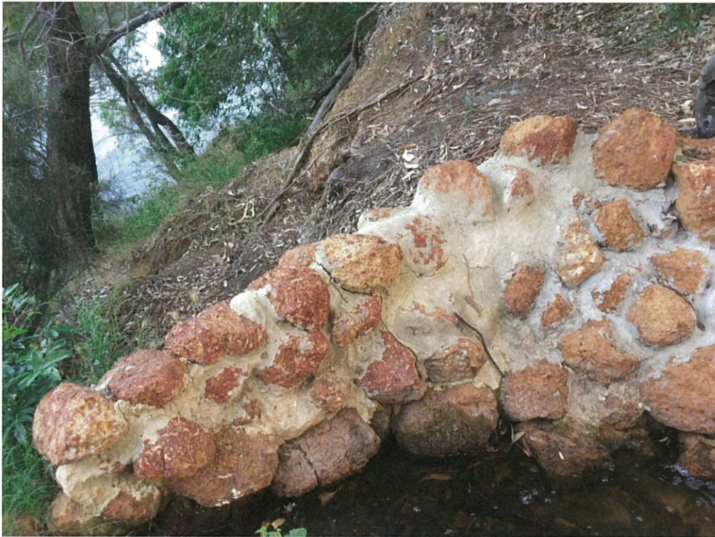
Photograph 3: Tension cracking within the existing structure.
