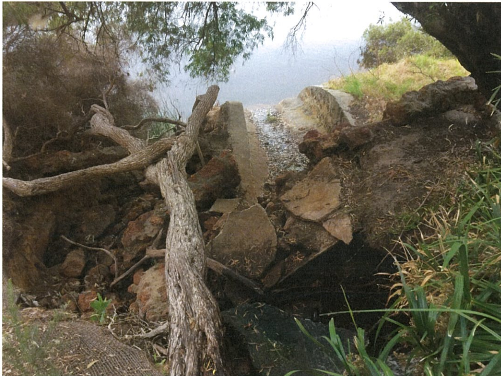
Photograph 1: Scour feature and collapsed 2 nd tier concrete structure.
