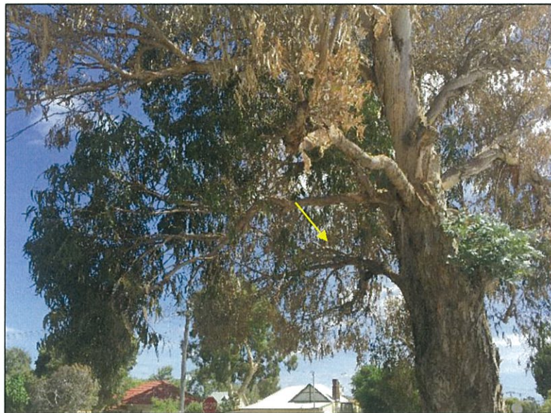
Figure 6. A number of live branch sections were visible throughout the crown and as such remedial works should be limited to monitoring only (no pruning to be undertaken), to assess the ability of the tree to produce new foliage; looking towards the northwest.
