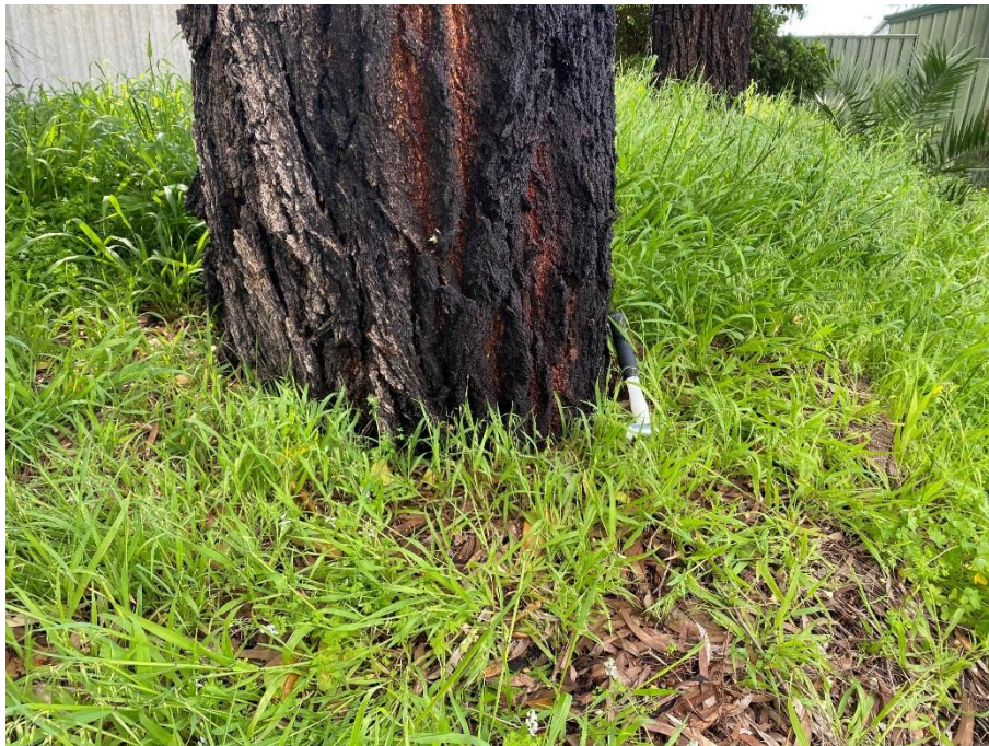
Figure 6. Adequate rootplate development was deduced however minor fill soil atop the original grade was evident; looking towards the northeast.
