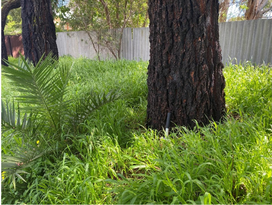
Figure 10. No significant trunk defects or wood decay was observed and sounding with a nylon hammer failed to return any tonal variations indicative of a thin residual trunk wall; looking towards the northwest.
