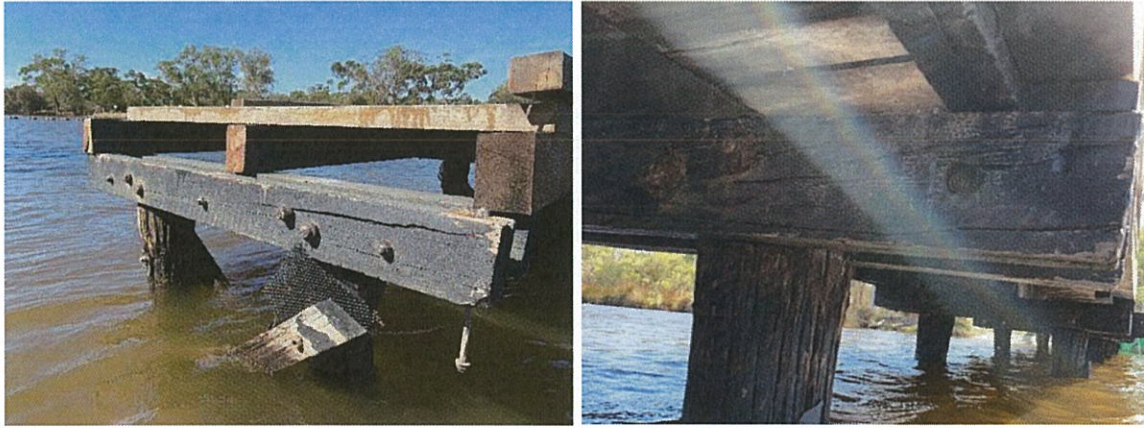
Figure 2.3 Half Caps – Poor Condition
