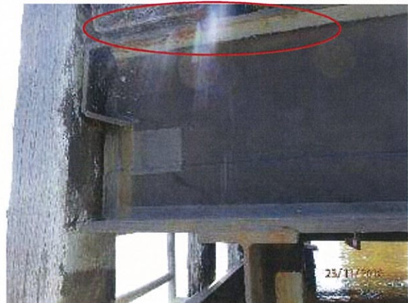
Photo 52 - Early spot corrosion evident to steel stringers on the top flange on external exposed faces. Note: Previous paint repairs/patches were evident.
