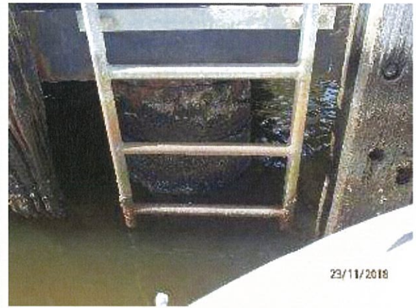
Photo 46 – Deterioration of galvanised coating and early corrosion on the bottom of ladder (in the tidal zone).
