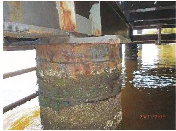
Photo 50 – Moderate corrosion evident to top of piles above current pile wraps.
