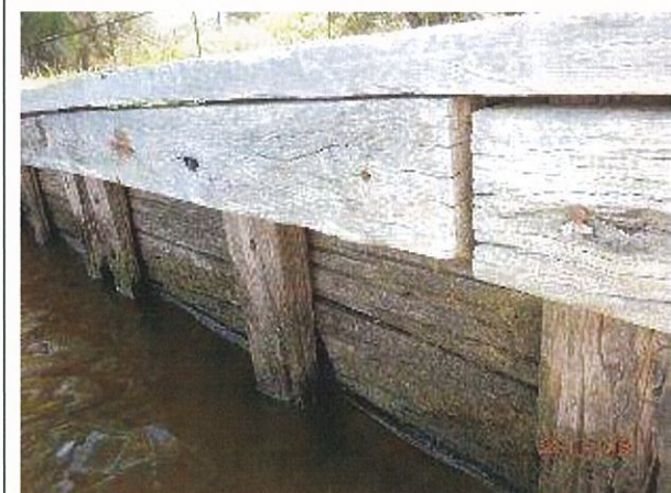
Photo 23 – Extensive weathering, splitting, section loss and rot evident to shore timber retaining wall on downstream side of jetty.
