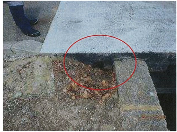
Photo 34 – Typical view of material loss at sides of jetty concrete slab connection with shore.
