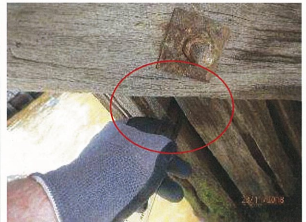
Photo 16 - Significant crack/section loss in timber pile on pier 2 with plastic ruler penetrating split across majority of pile diameter.
