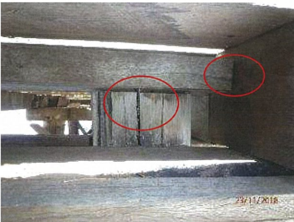
Photo 7 – Poor connection of timber stringer to pier, with split in timber at location of metal screws.
