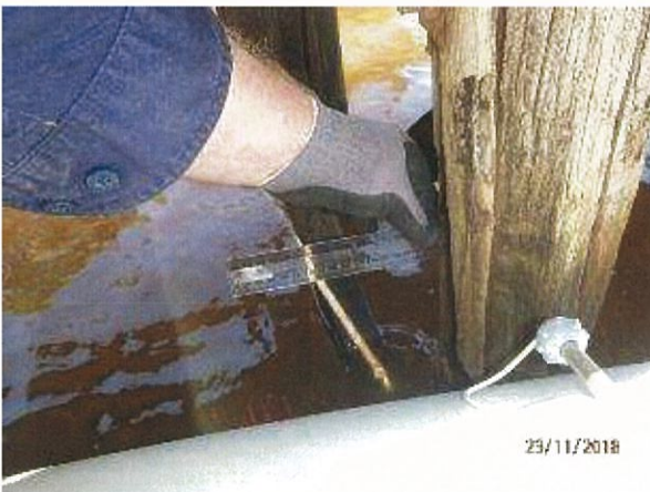
Photo 11 - Significant crack/section loss in timber pile on pier 1 with plastic ruler penetrating split across majority of pile diameter.
