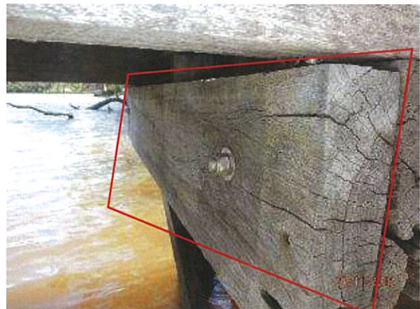
Photo 8 - Previous strengthening repairs to existing timber headstocks, by bolting of additional timber beam to side.
