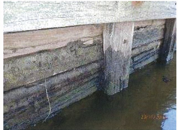
Photo 22 - Extensive weathering, splitting, section loss and rot evident to shore timber retaining wall on upstream side of jetty.
