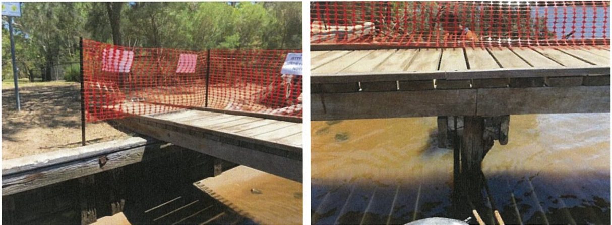
Figure 7: The two shoreside piles are smaller in diameter than the other four piles.
