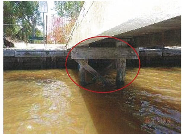
Photo 10 - View of near shore pier, with significant section loss/weathering on external surface of timber piles resulting in limited effective pile diameter supporting the jetty.
