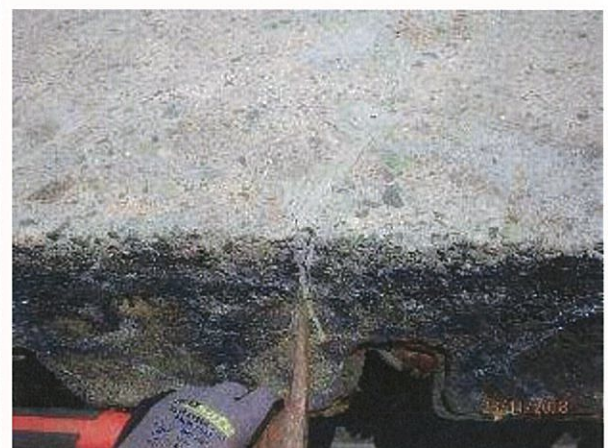
Photo 32 - Previous "V type" repairs to fine cracks in the concrete deck slab. Fine cracks in concrete slab appears to be full depth to the supporting sheet pile steel sections.
