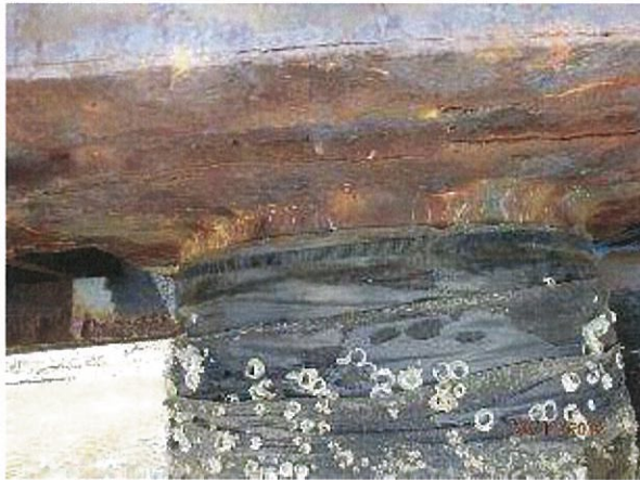
Photo 49 – Moderate corrosion evident to underside of the steel pile cap plates.
