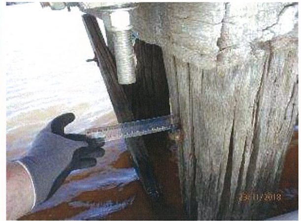
Photo 14 - Significant crack/section loss in timber pile on pier 2 with plastic ruler penetrating split across majority of pile diameter.
