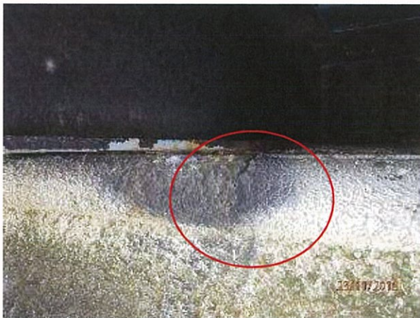
Photo 59 – A small crack was observed in the concrete seawall directly under the bearing area for the steel stringers.
