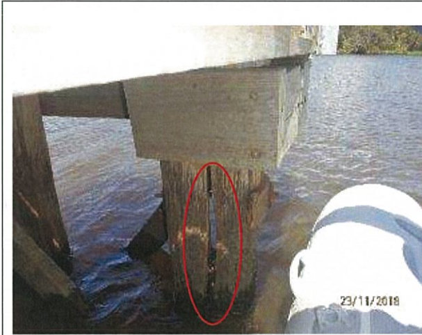
Photo 17 – View of end pier, with large crack with extensive weathering/section loss to internal section of pile.
