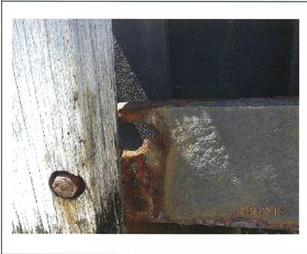
Photo 43 – Hole in steel water beam on the front of the jetty supporting the timber chafers.
