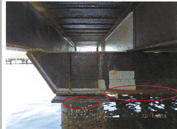
Photo 47 – Surface corrosion evident to top of steel pile cap plates and steel headstock beams.
