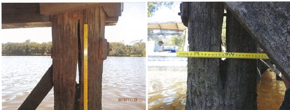
Figure 5: Shows vertical crack in outer western pile
