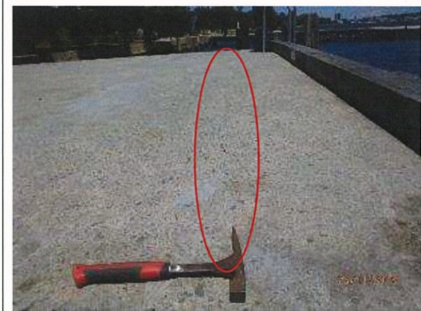
Photo 31 - Previous "V type" repairs to fine cracks in the concrete deck slab.
