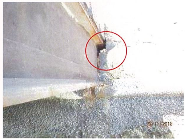
Photo 60 – A small hole was observed at the shore connection of the outside steel stringers and the limestone retaining wall.
