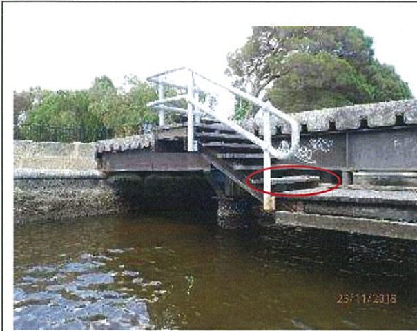
Photo 37 – Crack noted to lower timber stair tread.
