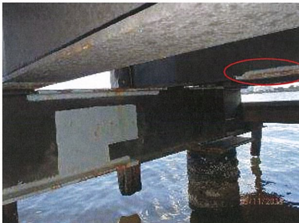
Photo 51 – Early spot corrosion evident to steel stringers on the bottom flange. Note: Previous paint repairs/patches were evident
