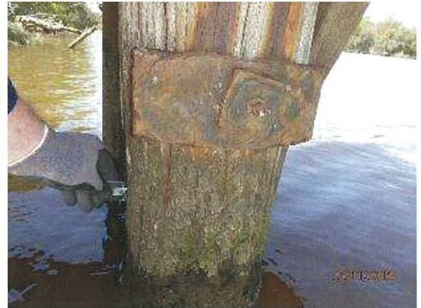
Photo 18 - Significant crack/section loss in timber pile on pier 3 with plastic ruler penetrating split across entire pile diameter.
