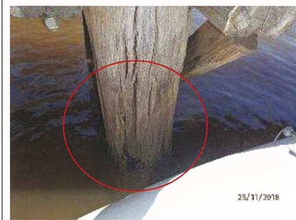
Photo 15 – Extensive weathering and section loss evident to external surface of timber pile on pier 2.
