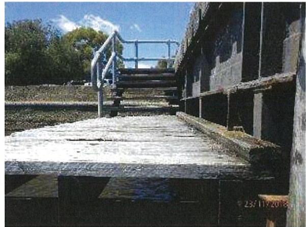
Photo 36 - Timber deck boards on the low-level platform appear very dry and require oiling/sealing.
