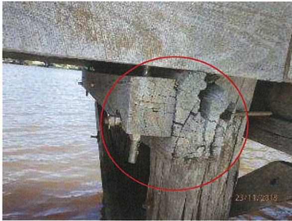
Photo 9 – Significant rot/section loss to original timber headstock beam and previous strengthening repairs to existing timber headstock, with additional timber beam bolted to side.
