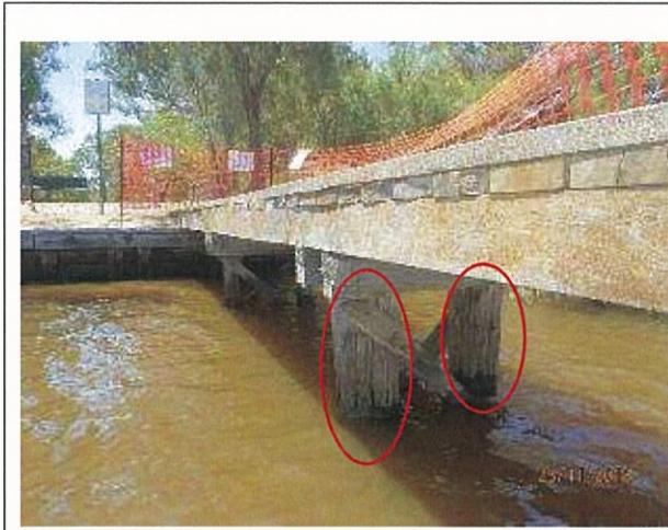
Photo 13 – View of central pier, with extensive weathering/section loss and large cracks/splits to external surface of timber piles.
