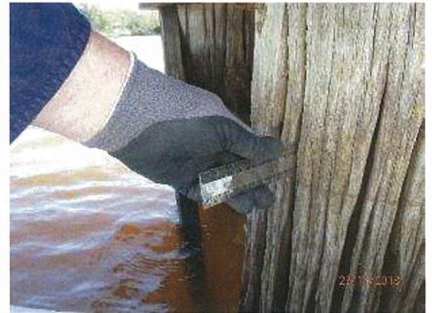
Photo 20 - Significant crack/section loss in timber pile on pier 3 with plastic ruler penetrating split across majority of pile diameter.
