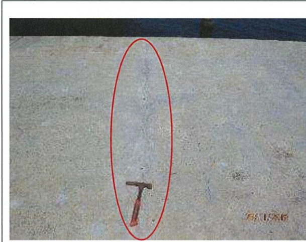
Photo 33 – Previous “injection type” repairs to fine cracks in the concrete deck slab.
