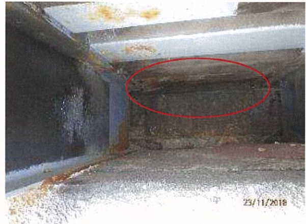
Photo 58 – Advanced corrosion was evident to the thin steel plate attached to the last steel sheet pile supporting the concrete deck (shore side).
