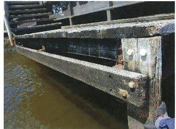
Photo 38 – The timber stringers (supporting timber deck boards), vertical timber chafers, and the timber waler beam on the low-level platform, all have evidence of significant weathering/splitting.
