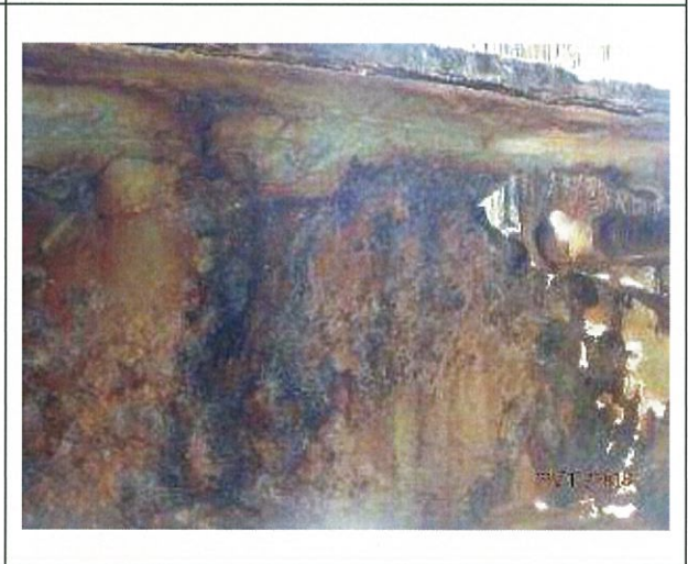
Photo 44 – View of steel water beam showing failed connection to timber chaffer and significant corrosion/section loss.
