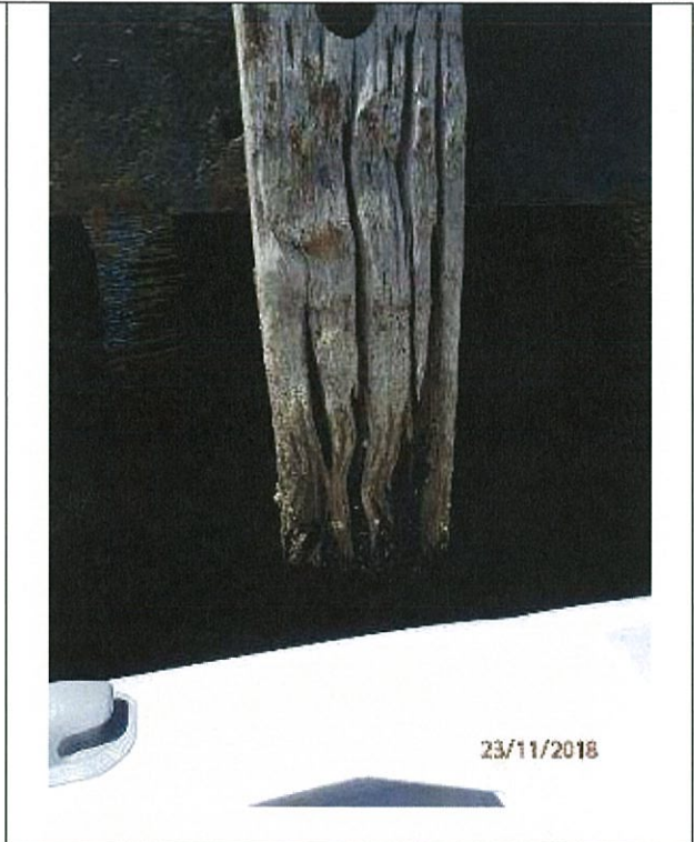
Photo 42 – View of the extensive weathering/cracks at the bottom of chafers.
