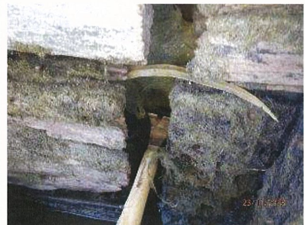
Photo 24 - Significant gaps were noted between longitudinal timber wall elements, exposing the filter cloth and potential loss of fill material from the shore.
