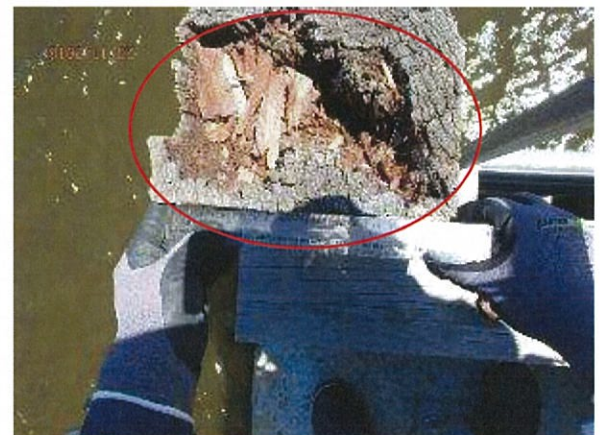
Photo 40 – Timber chafers unsealed at the ends with advanced rot/section loss in the top.
