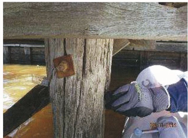
Photo 12 - Significant crack/section loss in timber pile on pier 1 with plastic ruler penetrating split across the entire pile diameter.
