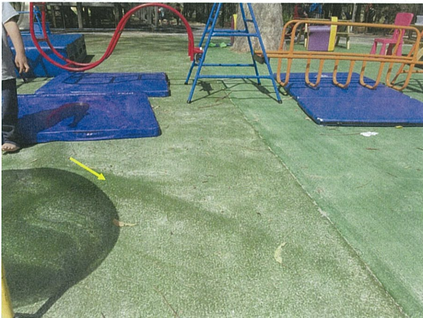
Figure 4. A tree root of approximately 70mm in diameter was evident on the northwest side beneath the synthetic turf at a distance of 5.2m (see arrow); looking towards the east.
