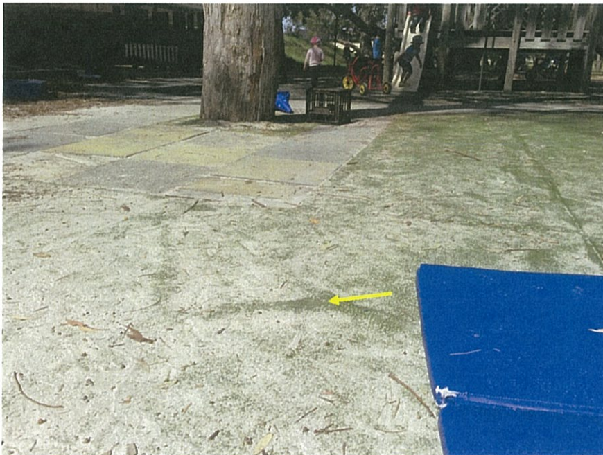
Figure 8. A root/ surfacing conflict was observed on the southwest side (see arrow) at a distance of 3.3m from the tree, with the root size estimated to be 20mm in diameter; looking towards the northeast.
