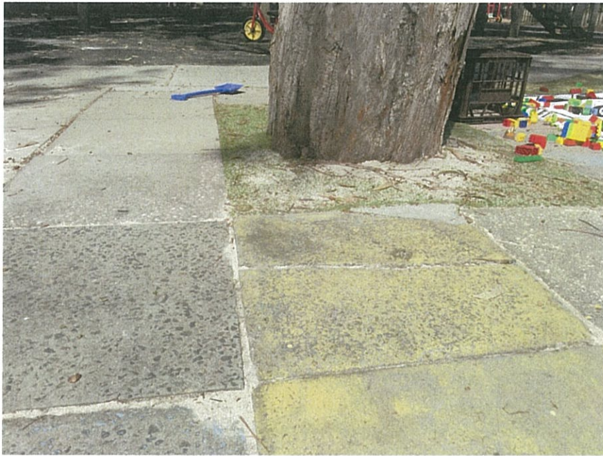
Figure 7. Concrete slab pavers were visible as the surface treatment with closer inspection revealing cracked pavers as well as displacement by approximately 10mm, typical where hard surfacing is located in close proximity to mature trees; looking towards the east.
