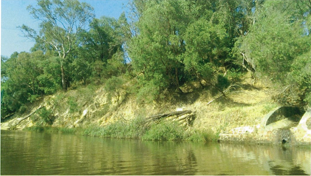
Photograph 5: (Right) Outflow structure. (Left) Recent collapse of several trees due to ongoing slope instability.
