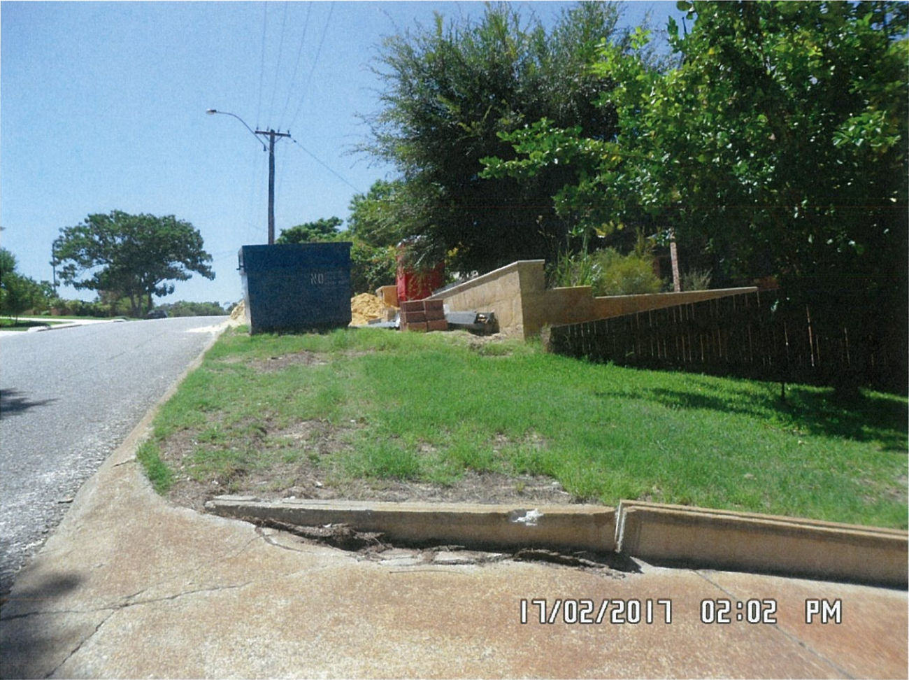
Photo of the crossover and the verge after being hit by the truck and before removing the retaining wall
