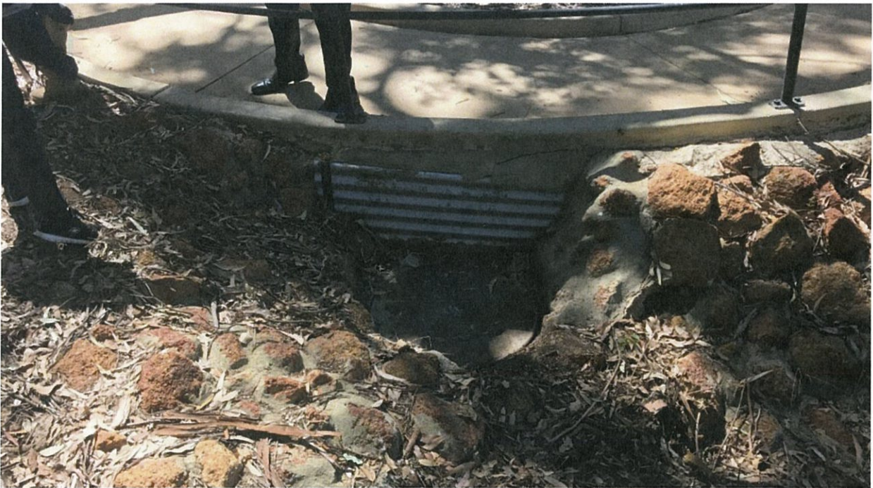
Figure 16 Image of cracked stormwater pit from the ground surface
