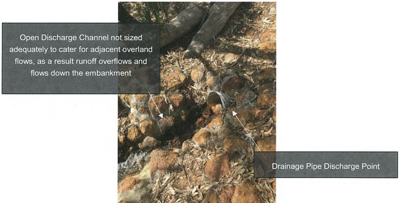
Figure 10 Pipe Discharge Open Channel
