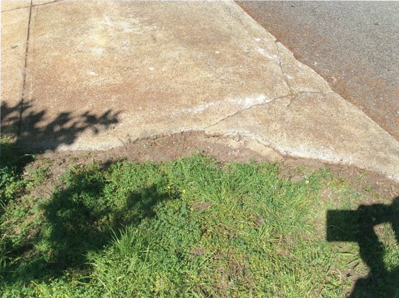
Photo of the crossover and the verge after being hit by the truck and after removing the retaining wall
