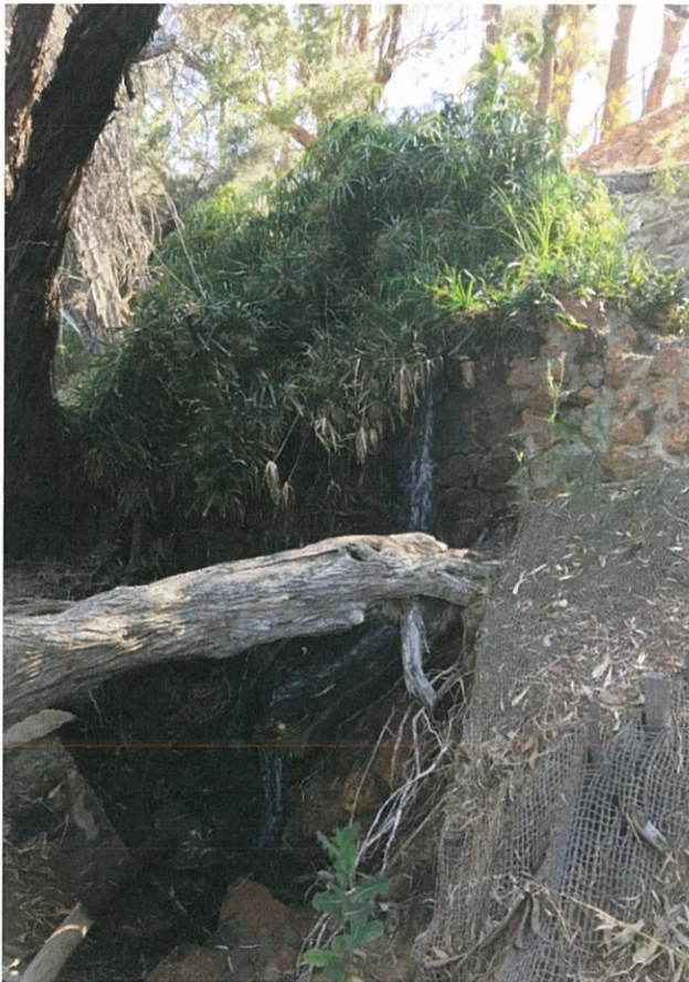
Figure 1 Degraded Spillway Structure
