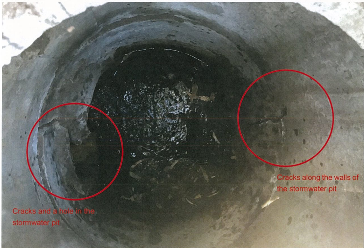
Figure 15 Image of cracks in stormwater pit that requires patching and sealing
