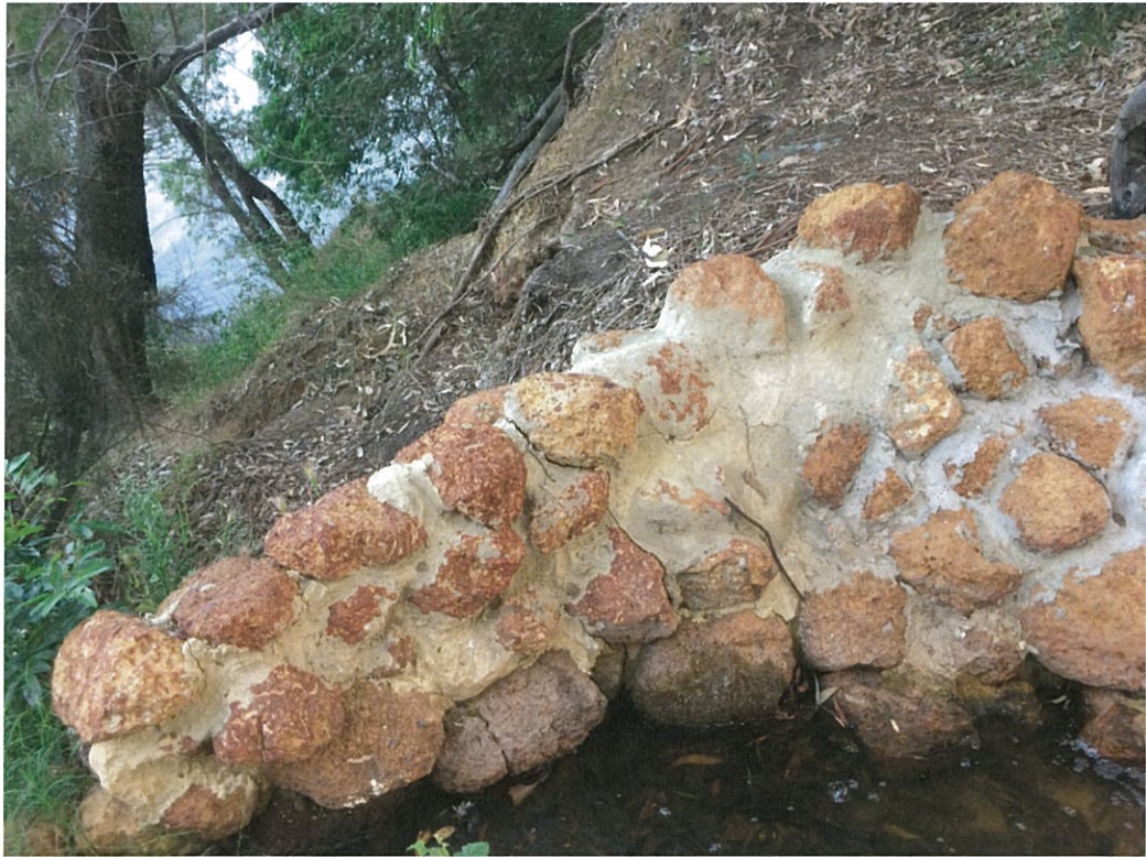
Photograph 3: Tension cracking within the existing structure.
