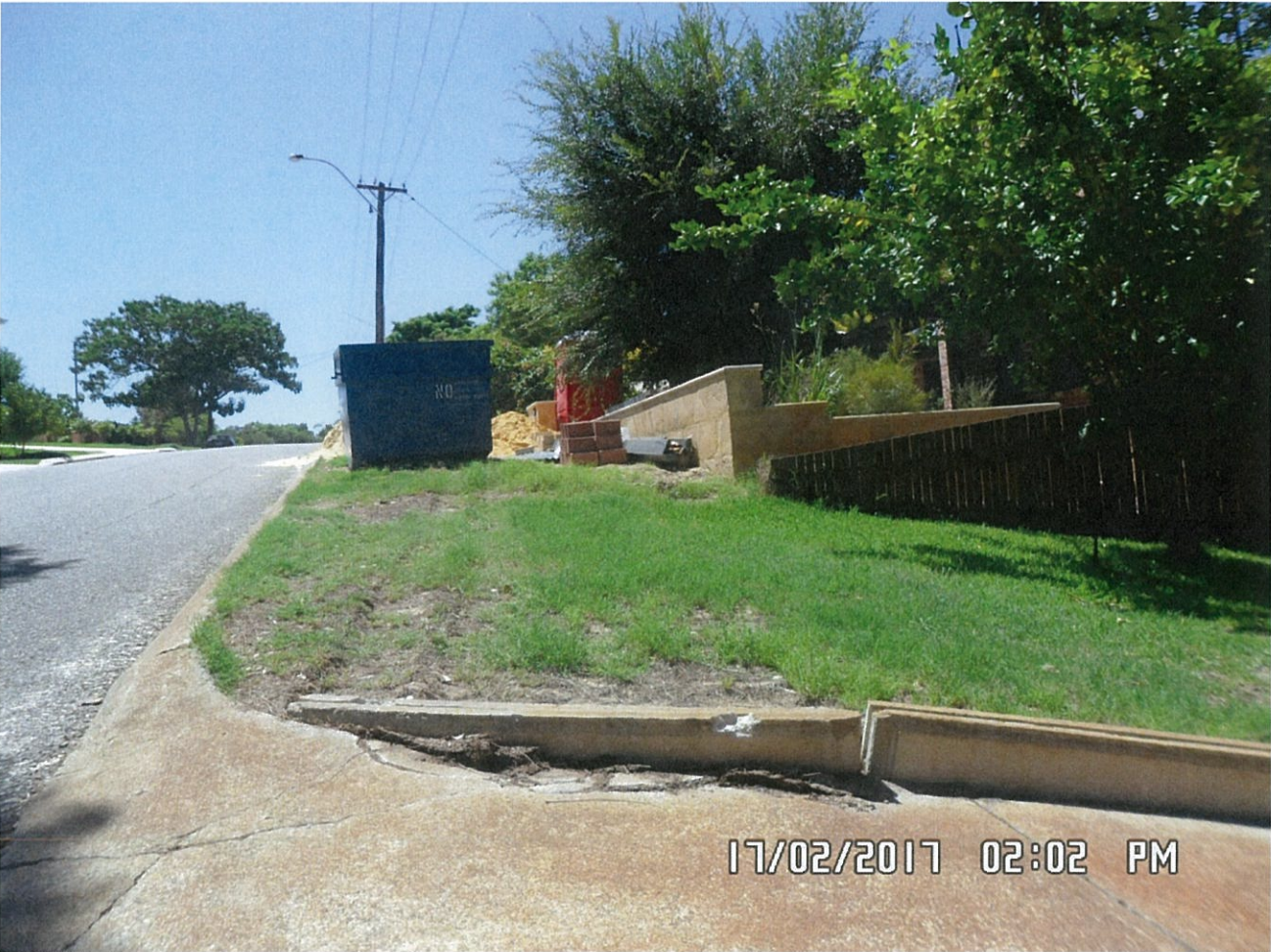
Photo of the crossover and the verge after being hit by the truck and before removing the retaining wall
