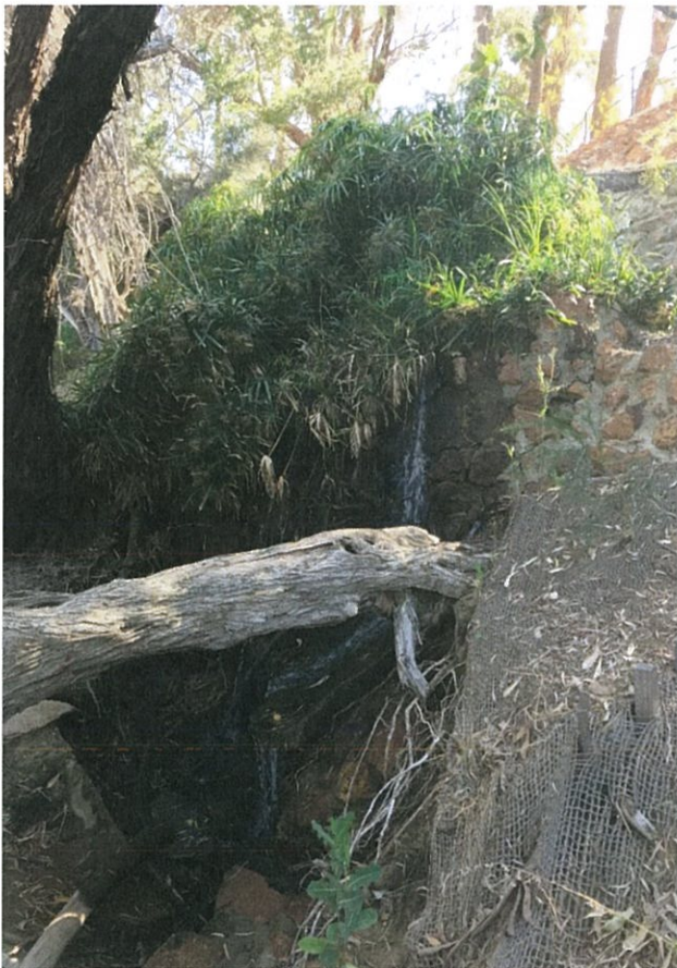
Figure 1 Degraded Spillway Structure
