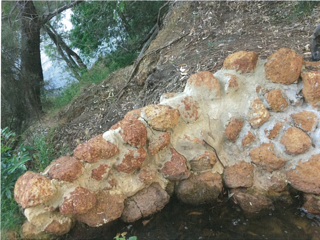
Photograph 3: Tension cracking within the existing structure.
