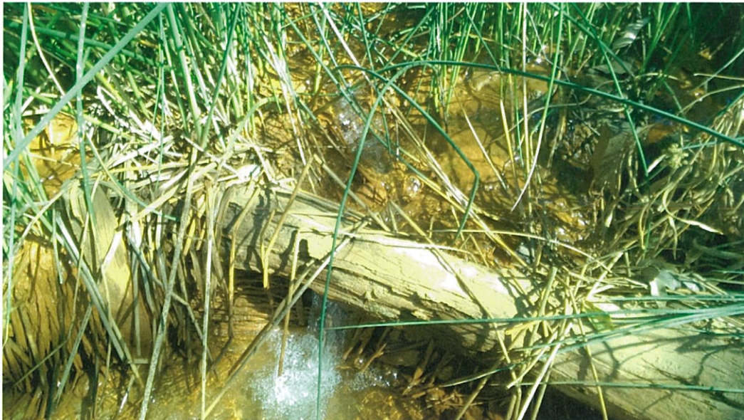
Photograph 4: Natural spring outflowing on the western river embankment upstream of the drainage outflow structure.
