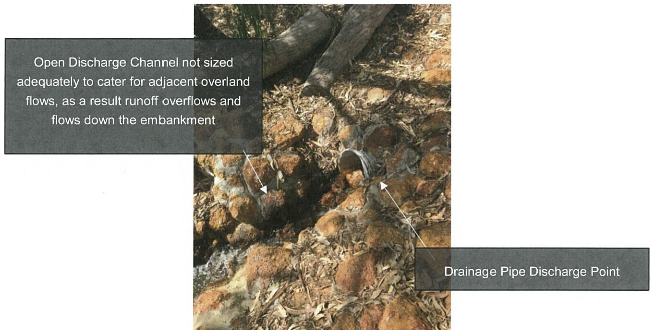
Figure 10 Pipe Discharge Open Channel
