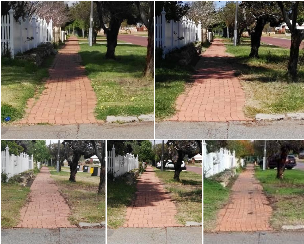
Figure 4: Glyphosate control on kerb line weeds, starting from top left: September 2020 (day of treatment), October 2020, November 2020, December 2020 and June 2021. Rhizomatous grass growing at the front of the brick foot path and adjacent kerb did not regrow.
